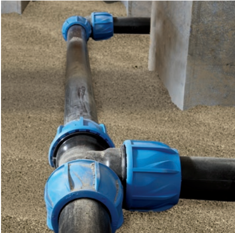
Water Distribution Lines
